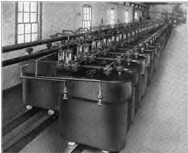
FIG. 137. Battery of I. O. C. generators.
